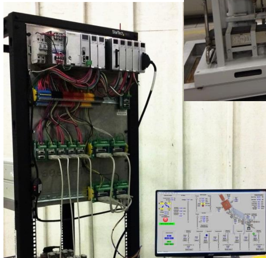
Industrial Accelerator Controls (Programmable Logic Controllers with PC interface)
