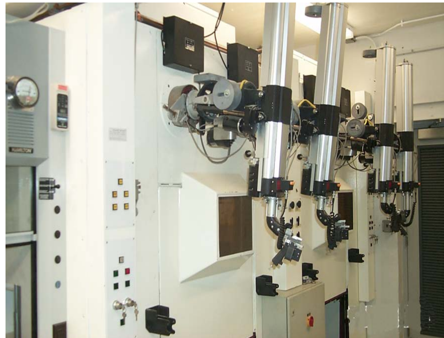
View of several processing hot cells
