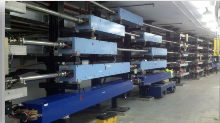
~500 Large Dipoles powered by >40 HVPS
