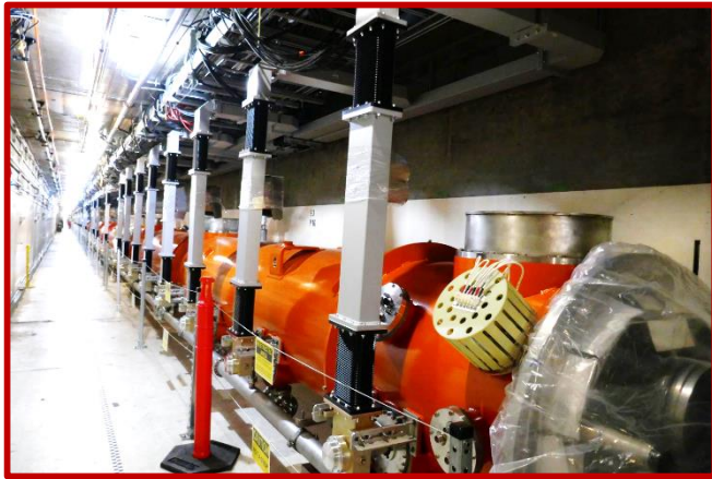
18/35 1.3 GHZ Cryomodules are in place. ~ one arriving per week
