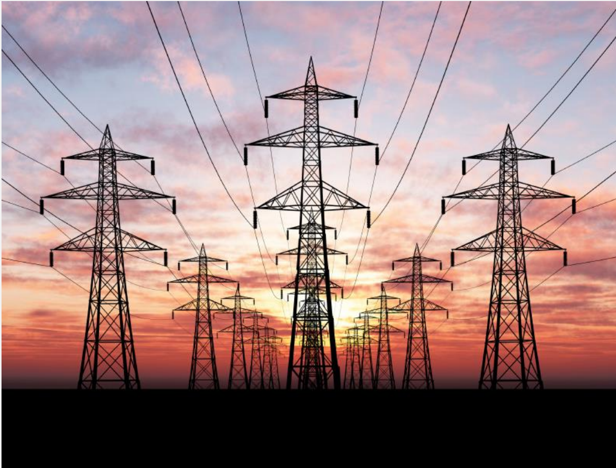
Figure X: Power transmission lines.
